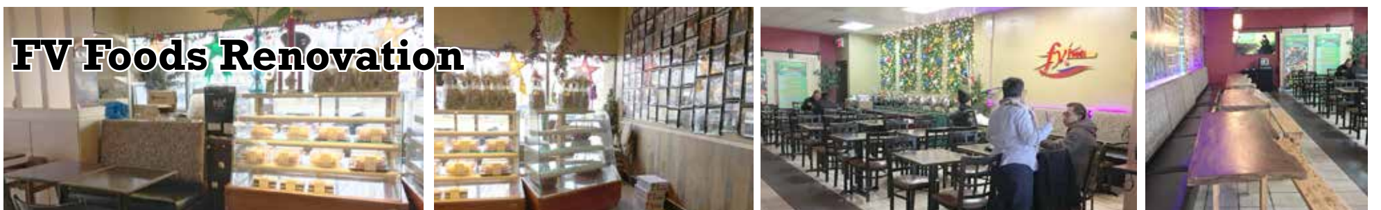
Fv Foods renovates Lawrence branch. Where there was a dining area beside the window, it is now replaced by a selling area. The dining area on the south side has been expanded by knocking down a wall and removing some rooms. Or I think a washroom. Benches have been added. They are thick wood and supported underneath.
